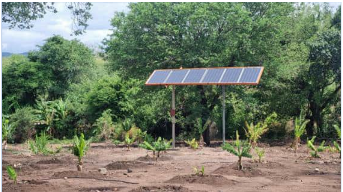
Figure 79: Solar Panel that Powers Four Water Sprayers to Irrigate the Crops at Titani Ranch
