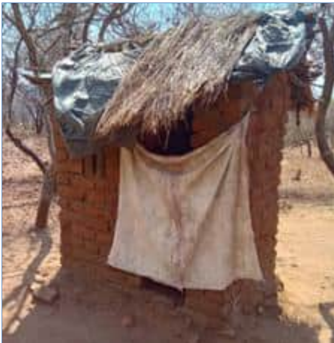
Figure 102: Typical Latrine (Feremu, Neno District)
