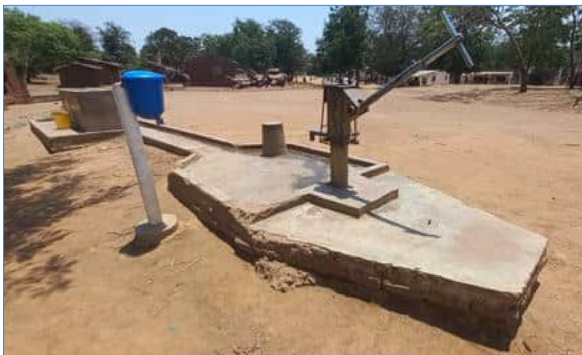
Borehole with Chlorine Dispenser
